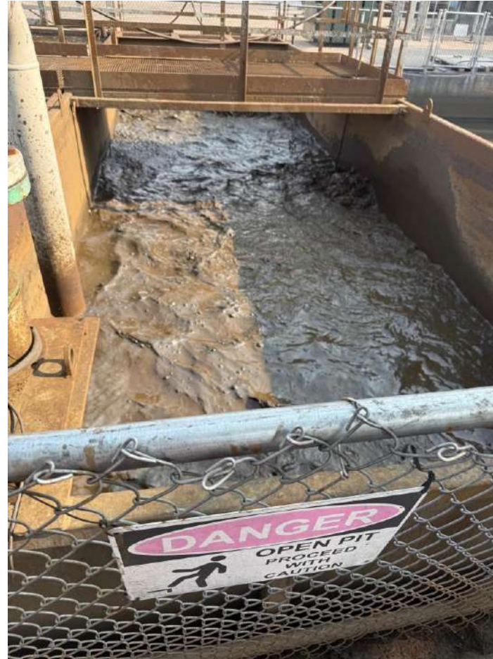
Fig 1. untreated waters flowing into the processing facility
